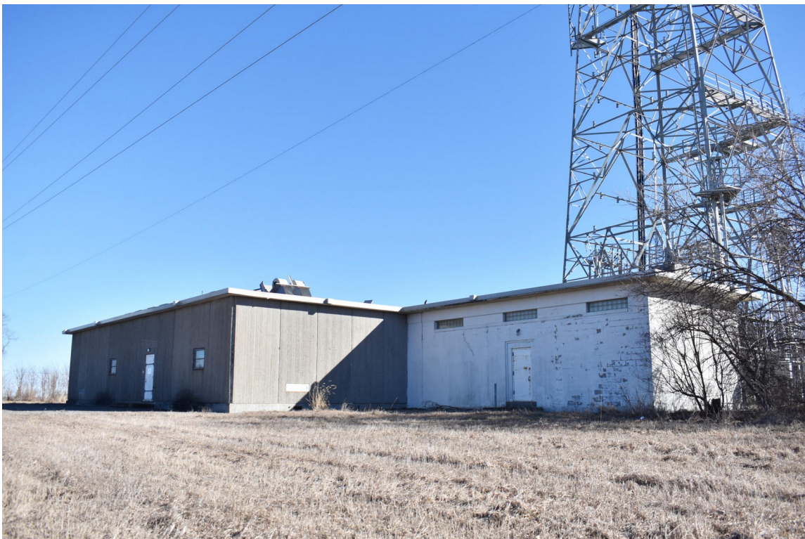
The original block building (c. 1953) is seen on the right, while the solid concrete “semi-hardened” addition is seen to its left.
